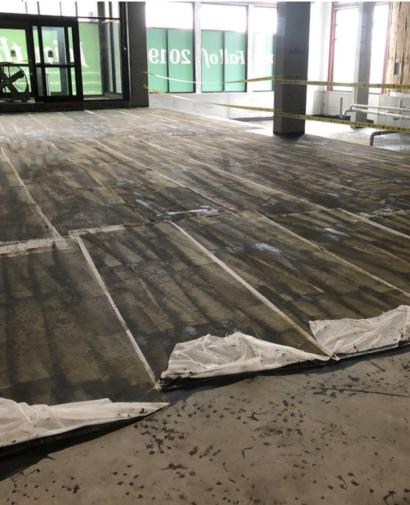
Installation of e.poly reinforcement fabric prior to the second application of e.roll.
