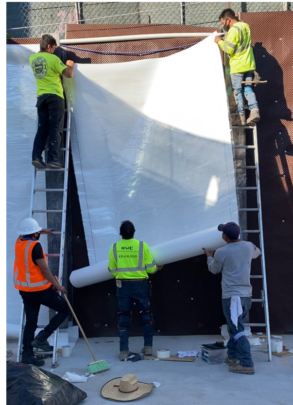
Installation of full 8 foot wide PreTak roll between back lagged soldier piles.
