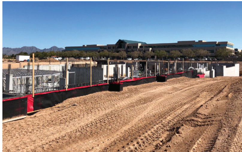
E.Protect terminated at grade.
