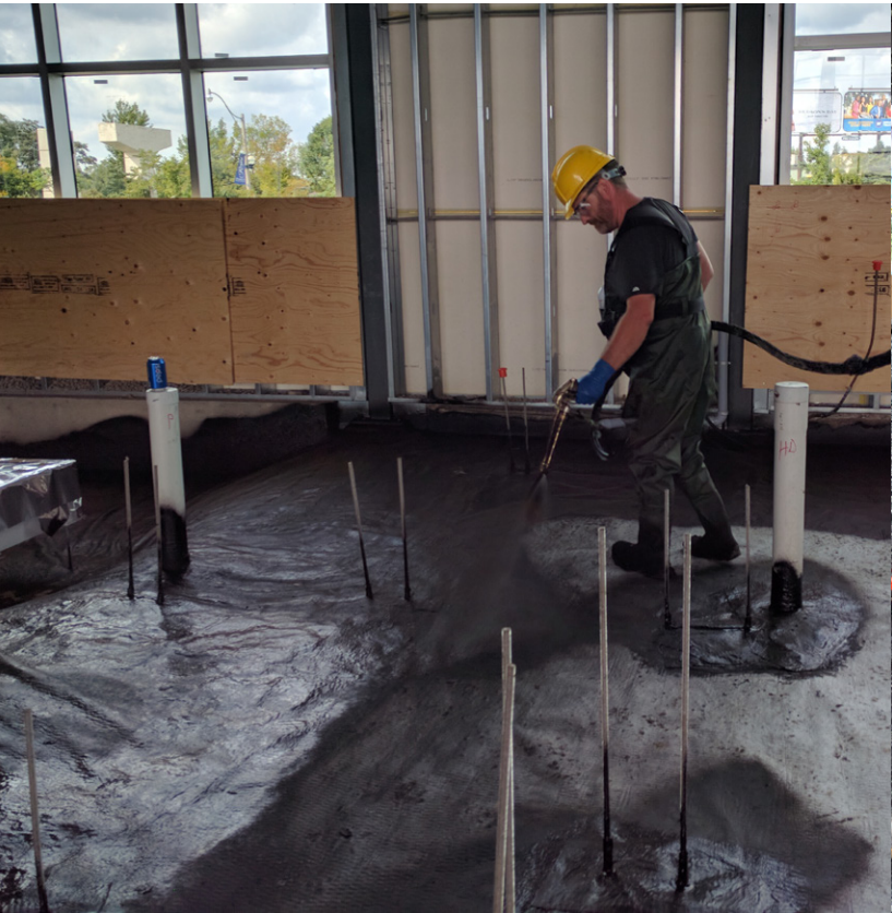
Along the north side of the building, e.spray is applied on top of e.base 205. Penetrations were reinforced with e.poly and e.roll, and allowed to cure before applying a bulk coat of e.spray to 60 mil.
