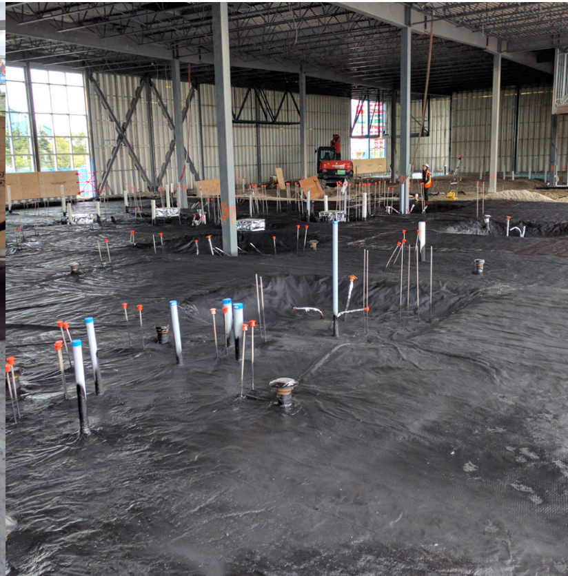
Looking northeast from the southwest corner. The first half of the building was completed with a bulk coat of e.spray to 60 mil. The material will be allowed to cure and then smoke-tested before application of e.shield 205.
