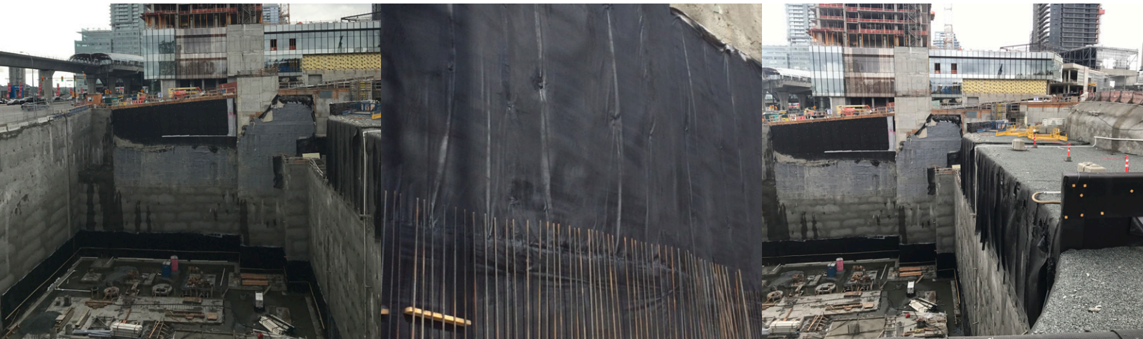
Looking over Tower 3 excavation. Here, the first lift of EPRO is being installed
